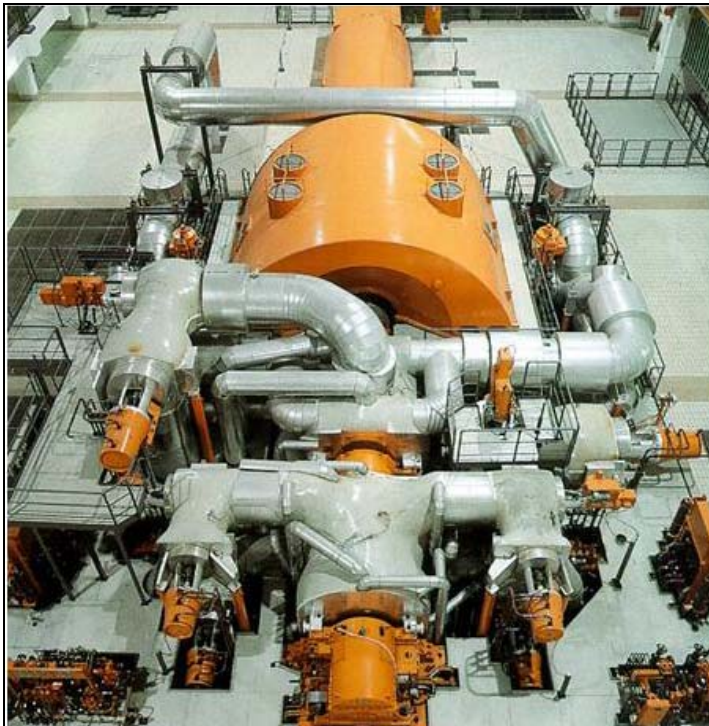
Figure 2.1: Modern steam turbine of a coal-fired power plant [165, NWS, 2001]
