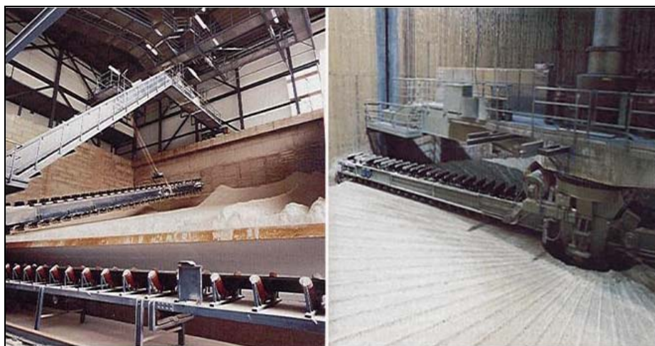
Figure 4.23: Closed gypsum storage facilities [94, Umwelt + Technik, 2000]
